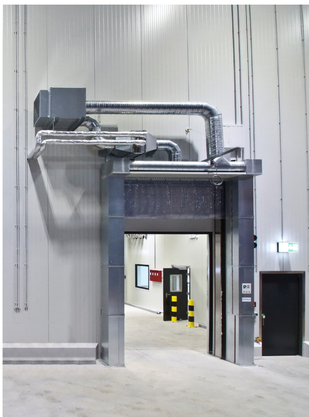
DSBLOCK + HEATER (Glycol)
