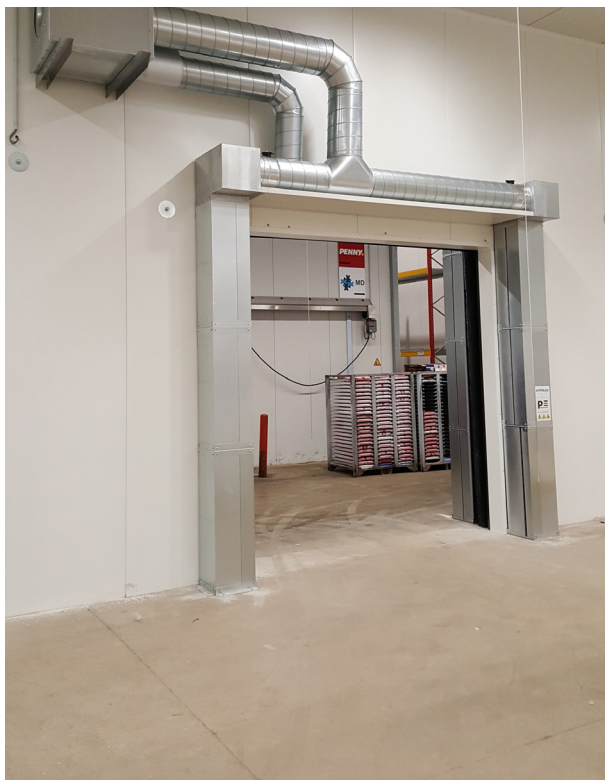
DSBLOCK + HEATER (Electrical)
